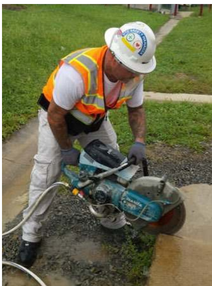
A construction worker using a handheld power saw with an integrated water delivery system.
