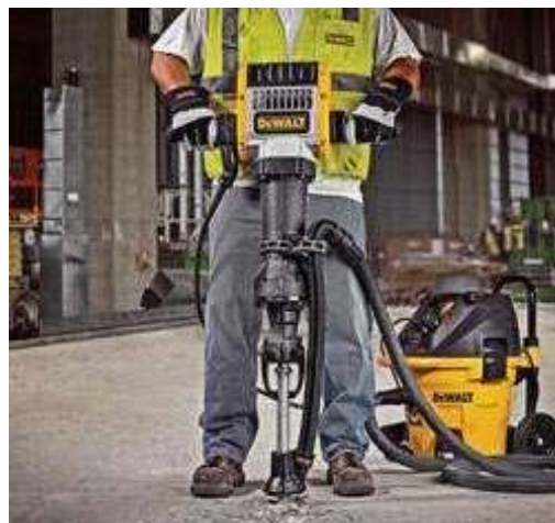
Jackhammer equipped with VDCS. Shroud around hammer connects to the vacuum on the right.
